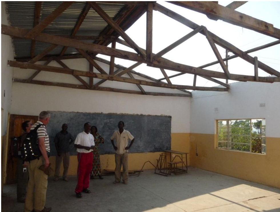
Figure 4 Damage to a classroom roof
